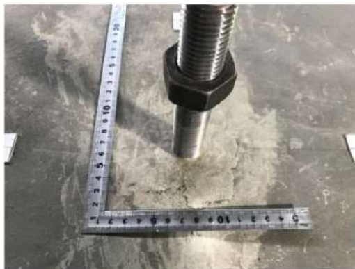
(ひび割れ箇所除去前)
